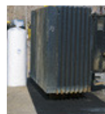
Ideal underneath leaking transformers.
