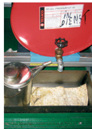
OP pads under oil cans & drums to catch small drips.
