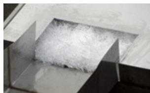
Filtering of waste water before discharging into water discharge area.
